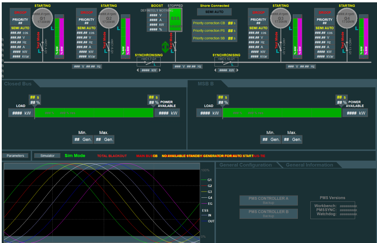
Figure 38: HMI for the Energy Management System (EMS) from Vard Electro
